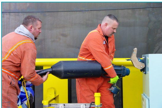
Longshore plugging TOTE vessel into shore power
